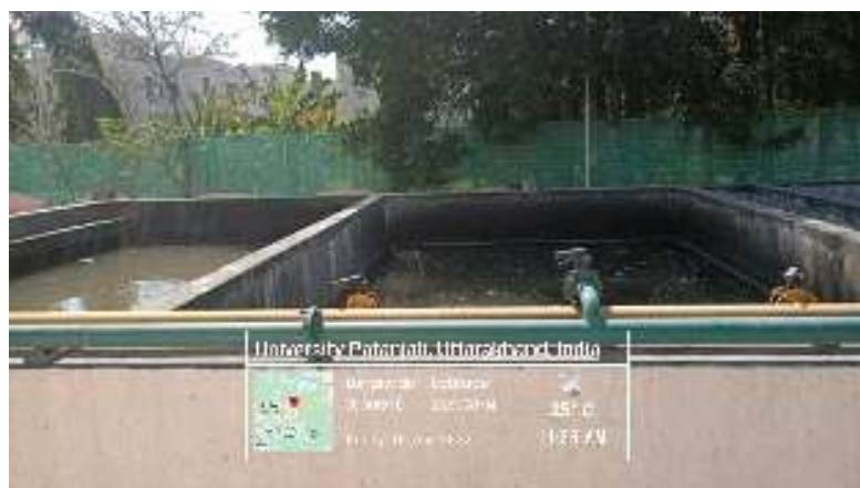
Sewage Treatment Plant (STP) during recycling waste water
